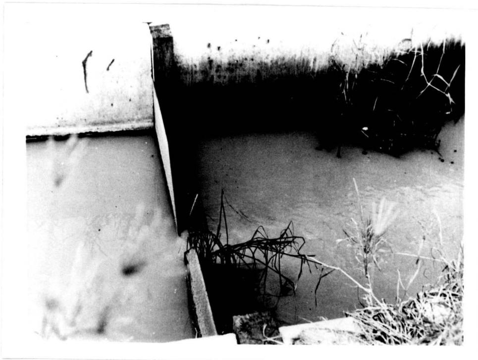
Plate 14 Treated Water Flow Through an Overflow Weir into Klong.
