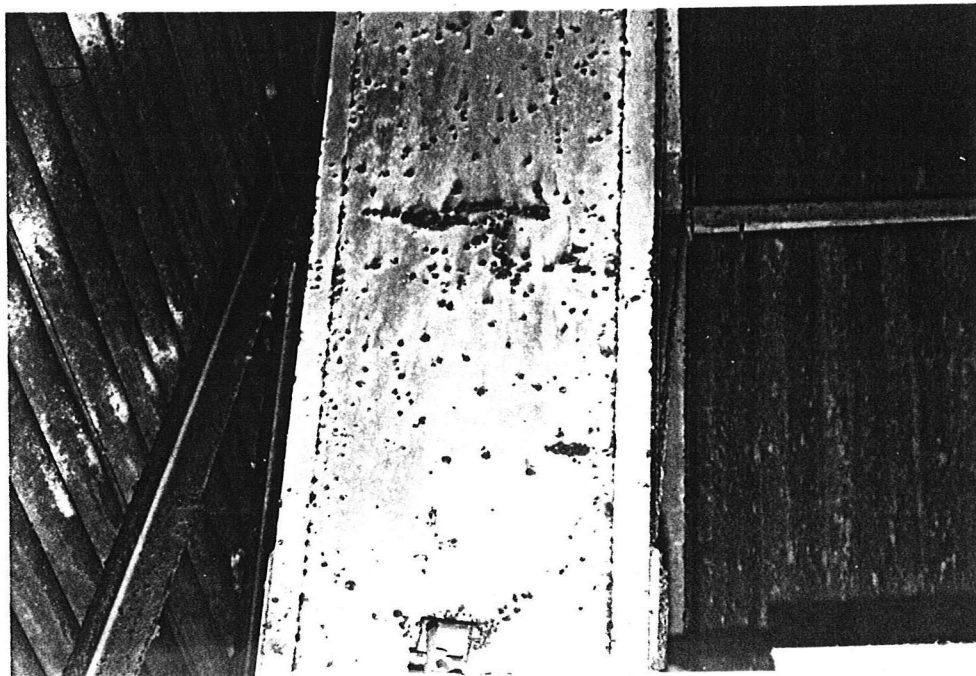
Fig. 2 Severe blistering in steel structure
