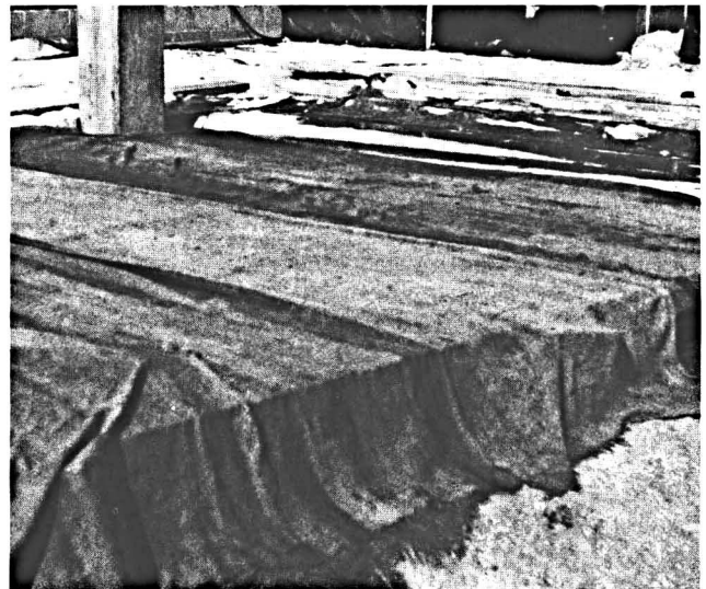
Fig. 32. One method of wet-curing is to completely cover the surface with wet burlap, keeping it continuously wet during the curing period.
