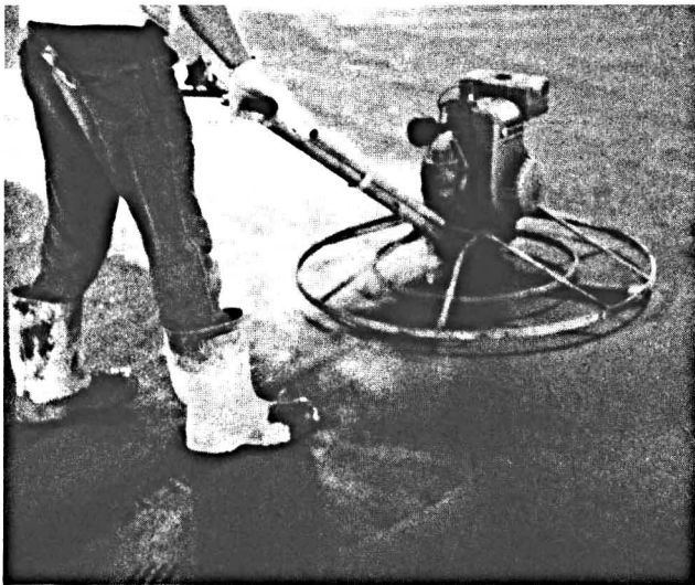
Fig. 31. Power troweling is begun when excess moisture brought to the surface by floating has evaporated and the concrete is not sticky. Two or more passes frequently are required.
