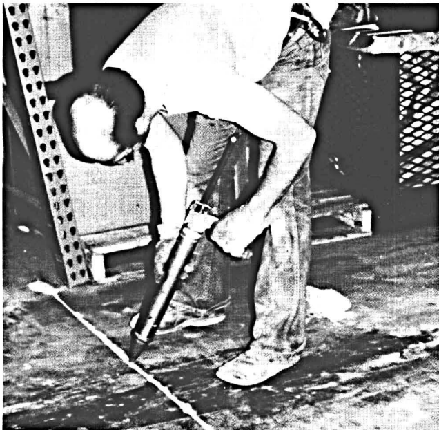
Fig. 35. Joints and cracks that move can be refilled with flexible sealant.
