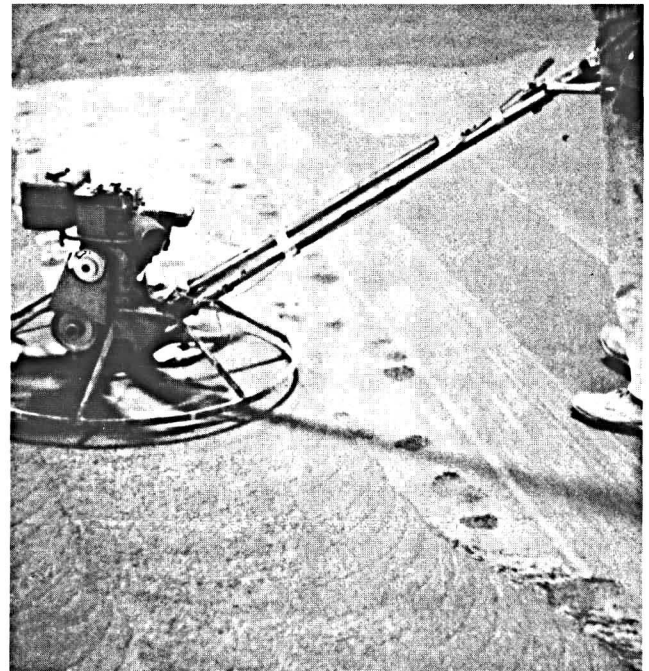
Fig. 28. Floating is begun when the water sheen has disappeared and the weight of a person leaves only a slight indentation on the concrete surface.
