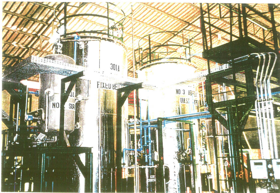
Photograph of Pilot Plant IN Thailand
