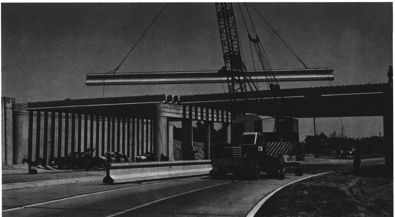
Fig. 17. Using precast-prestressed concrete girders facilitates construction and minimizes interference with traffic. This photograph shows precast-prestressed girders being erected to carry the Garden State Parkway in New Jersey over U.S. 322 and U.S. 40. Design: Gannett, Fleming, Corddry & Carpenter, Inc., Harrisburg, Pa. Construction: S. J. Groves & Sons Co., Woodbridge, N.J.
