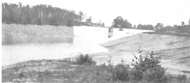
Figure II-25—Buried Asphalt Membrane Lined Reservoir, Rutland, Vermont. (Reservoir partially filled—note marble slab cover on dam section)
