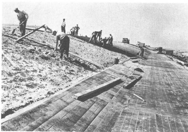
Figure IV-1—Workmen Placing a Sand Asphalt Course on a Sea Dike in Holland
