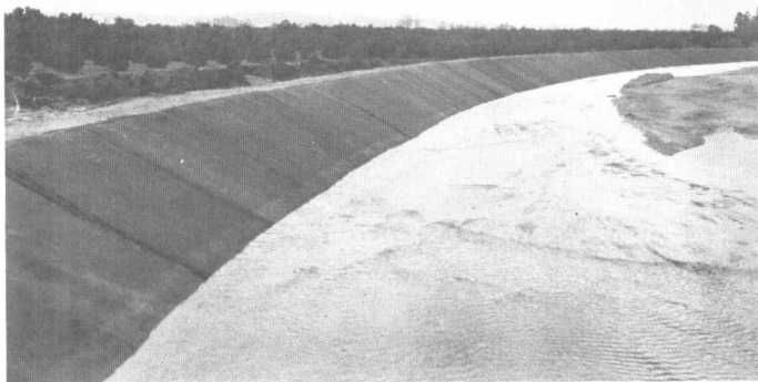
Figure II-16—River Size Storm Channel, Bottom Unpaved
