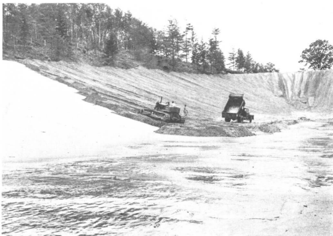
Figure II-23—Placing Cover Over Membrane by Dump Truck and Dozer, Rutland, Vermont Reservoir
